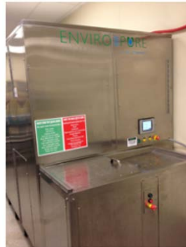
Figure 1.2. The EnviroPure waste disposal system located in Randall Dining Hall
