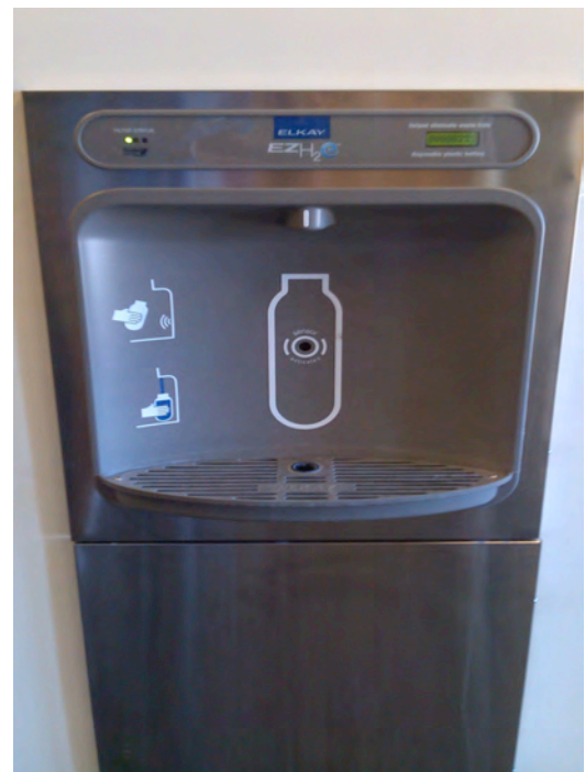
Figure 7.4b. Location: ETC Refill station with motion activated sensor and display showing number of 12 ounce bottles saved by refill station.
